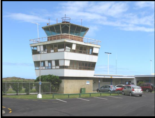
The Control Tower, now in need of restoration. Some glass panes have already been removed.
