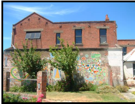
Ridgway Street façade of building first used as Solicitor’s office (B5 21bm)
